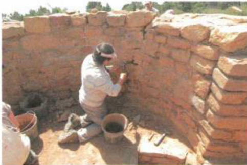
An intern with the Ancestral Lands Program meticulously replaces the surface layer of mortar between stones, called “repointing,” to weatherproof precious walls.
